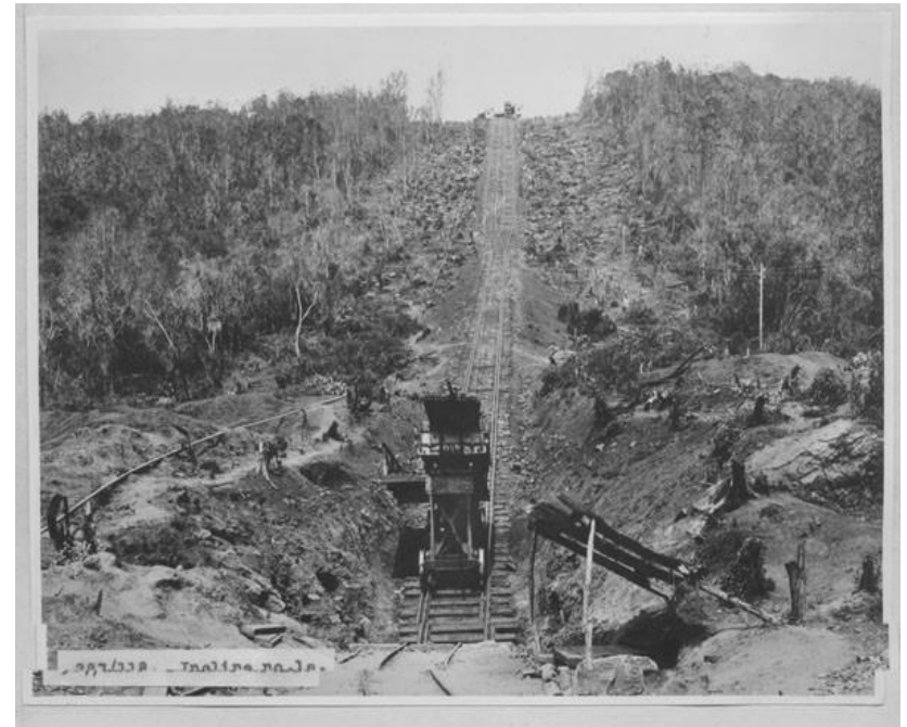
The steep inclines paused a major challenge to the contractors. A specially made Engine to carry construction materials down the inclines.
